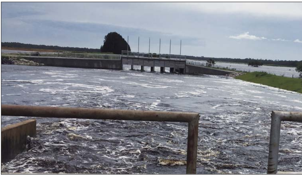
Figure 7. New Control Structure 1 viewed from upstream (old control structure) during Tropical Storm Hermine.
